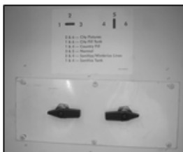
Fig. A Water Valve Controls
